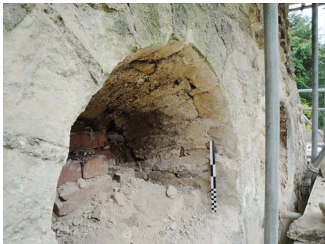
Window (D10). East face after removal of 19th-century blocking to the upper part. Note the rough nature of the rendered to the splayed part of the head and the fact that the render spalls over the dressed Caen stone.
