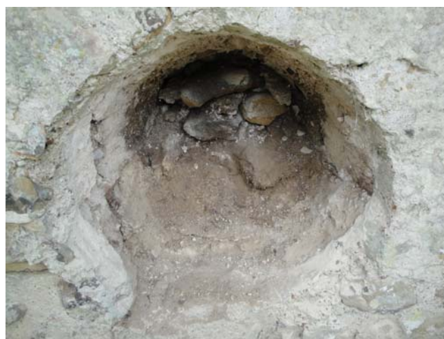
Circular window (D12) viewed following removal of the eastern skin of blocking on 1/8/2012.
