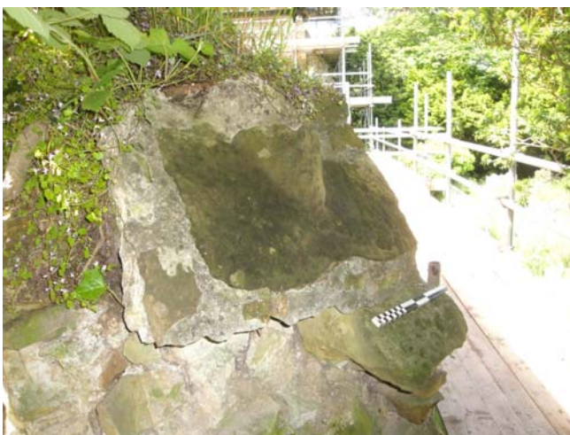
Remains of finial on offset of Buttress (G6).
