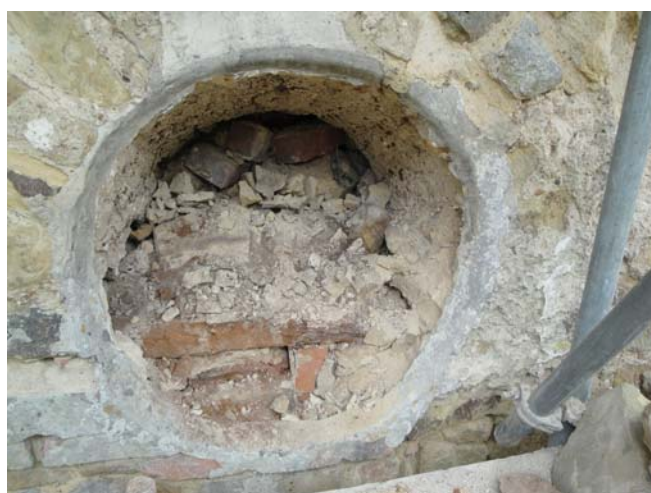
Circular window (D13) following removal of external blocking, 1/8/2012. Note the high-level timber lintel over blocked doorway D7/D11 and the way the face of the lintel is set back and the brickwork over the doorway's low-level lintel (not visible in photo) is roughly curved in order to maintain the window's outline as an antiquarian feature within the face of the wall.
