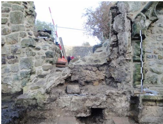
Window G2. Internal face after removal of pulpit showing dressed splayed quoins, cut-off phase-4 cill and phase-5 downward extension.
