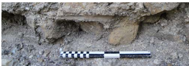
Window G2. Rear (northern) edge of phase-5 window cill visible as an impression in the mortar.
