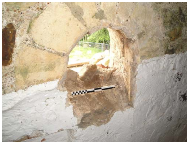
Window (D10). West face after removal of 19th-century blocking to the upper part.
