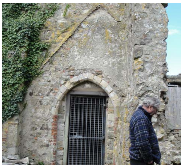
South wall of tower showing doorway (A2) and roof scar of porch (A5).
