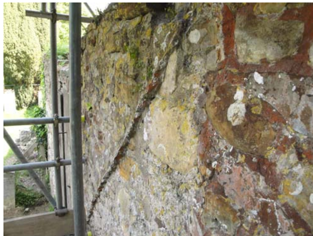
Mortar listing (F3) showing the line of the vestry roof.
