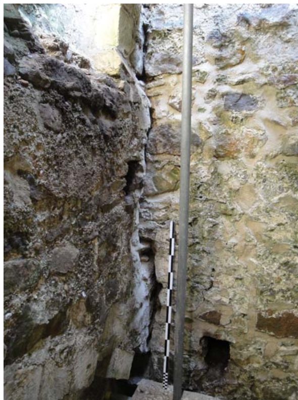
Block-bonded straight joint D43 rising from arch D25 to chamfered offset at cill level of openings D18 and D19.
