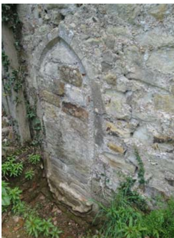
Blocked doorway (F7).
