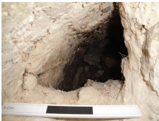
Circular window (D12) showing shuttering marks on interior of window head after temporary removal of a blocking stone.
