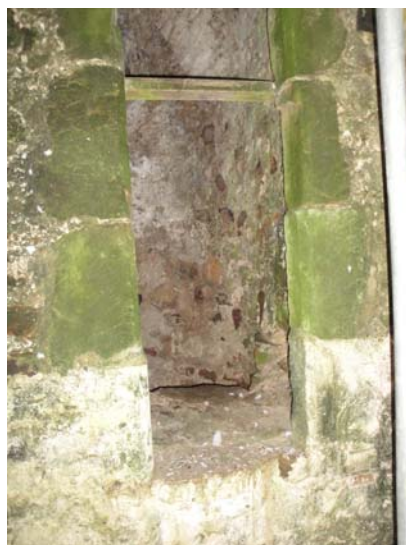
Base of doorway (C13) showing where the cill has been lower by the depth of one block.
