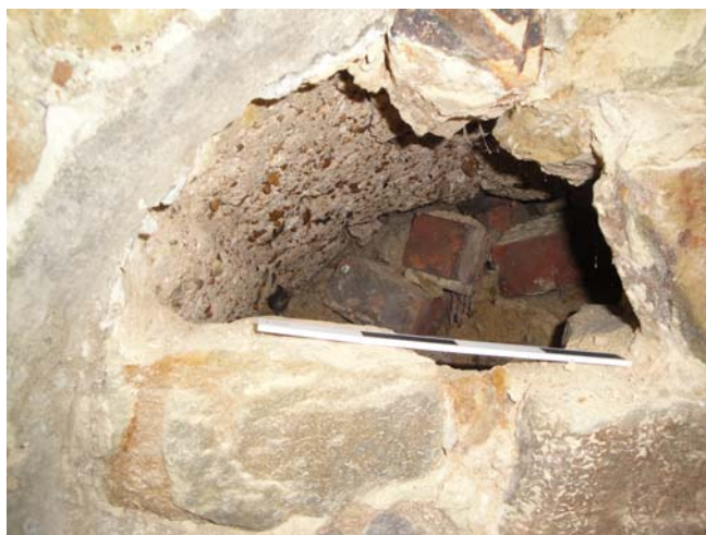
Circular window (D13) showing shuttering marks on interior of window head after temporary removal of a blocking stone.
