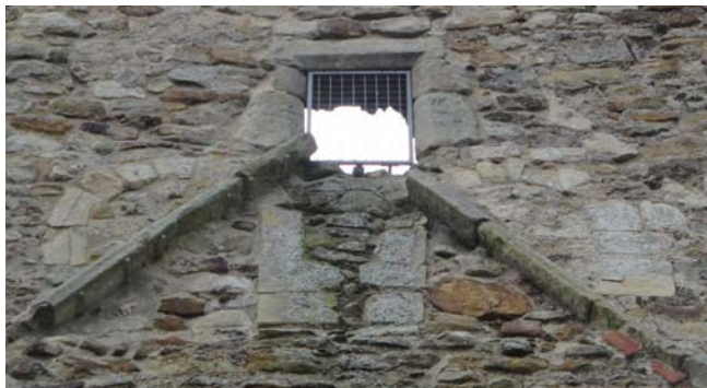
Roof weathering (D17) and blocked 'window' openings (D18 and D19).
