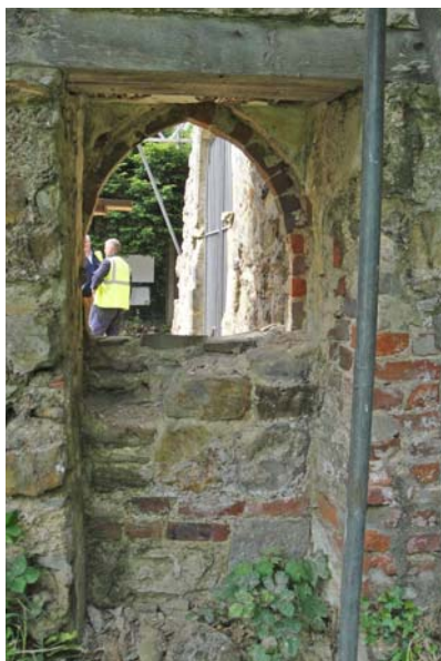
Rear arch of intruded doorway (F2) leading from nave into the 19th century vestry.
